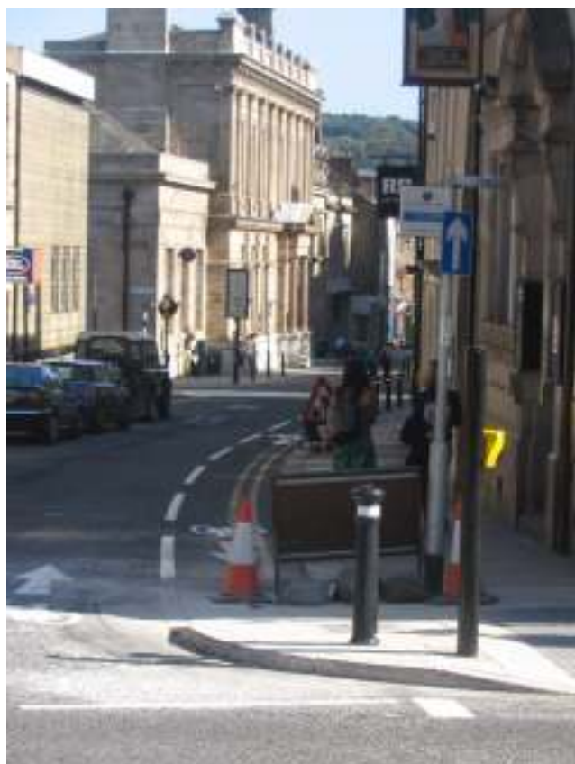
Cycle contra-flow lane at top of Upper Church Street under construction. This has now been completed, with a toucan crossing over China Street to the Judge's Lodgings.
